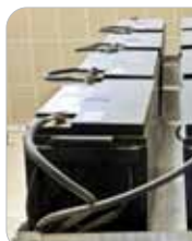
Industrial Battery Charging
