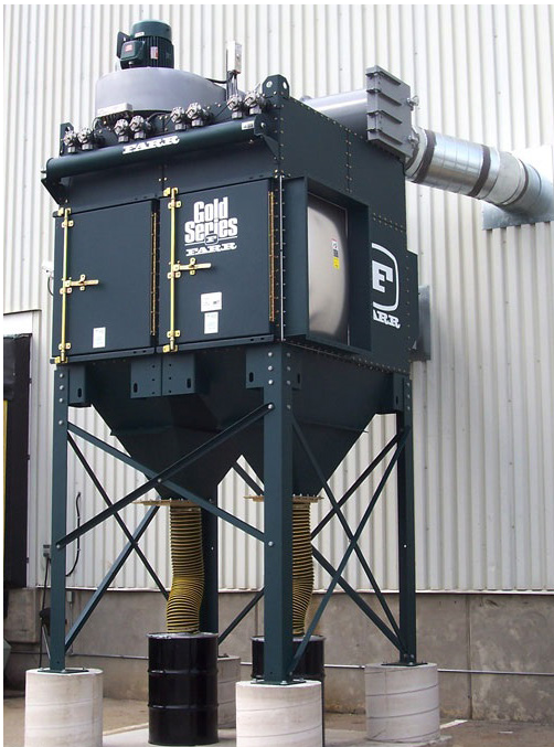
Dust collector at a pastry processing facility.
