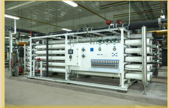
Built: 2008, Capacity: 3 MGD
