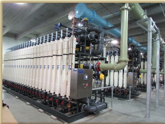
Built: Stage 1-2012 & Stage 2-2014 UF Capacity: 7.5 MGD, RO Capacity: 3.1 MGD
