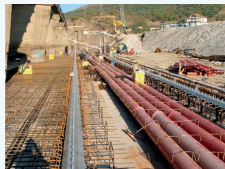
Anchor rails and pipe system
