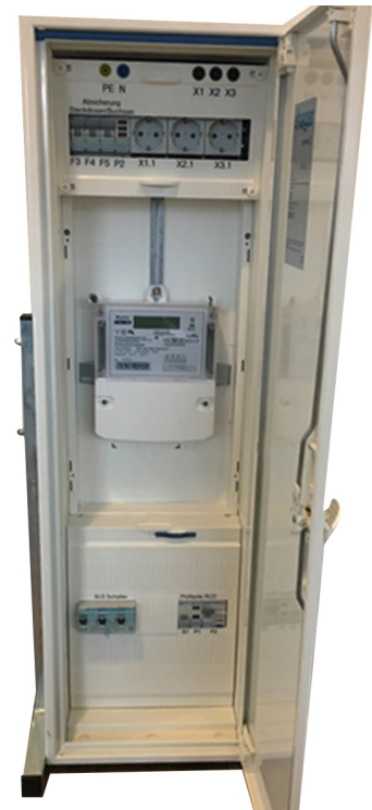
Figure 3: Typical metal cabinet for meter installation (normally attached to the wall). LoRa-enabled meter in the center.
