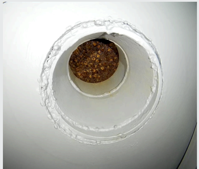
Storage tank nozzle
