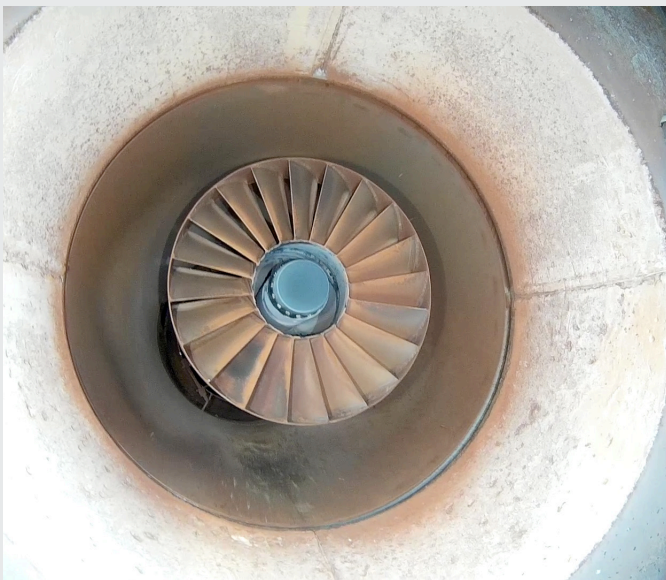
Burner in F3800 boiler
