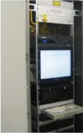
Fiber-optic control panel
