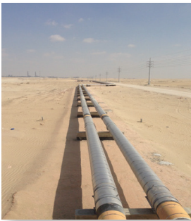
Engineered "Thermally Isolated" Pipe Supports and Anchors
