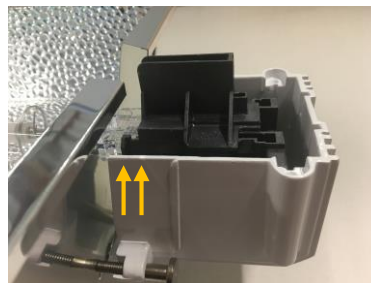
Lamp holder improperly closed
