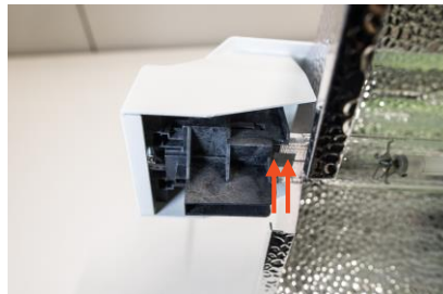
Lamp holder improperly closed
