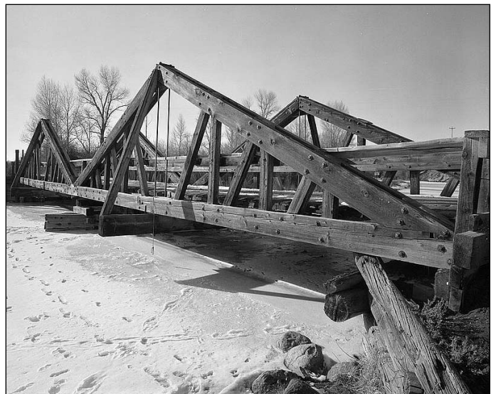
A wooden truss bridge over a frozen river in Wyoming. Photo courtesy of the Library of Congress.
