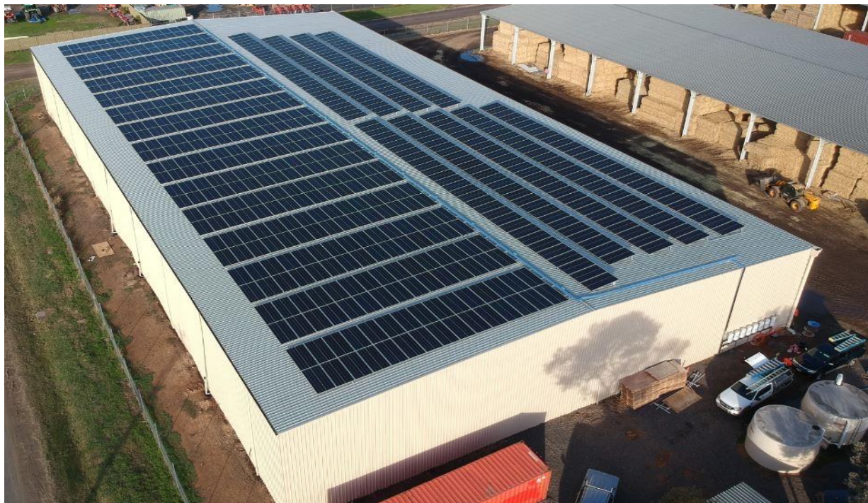
Above: Wingara's existing 275kW Epsom Solar Project Installation.
