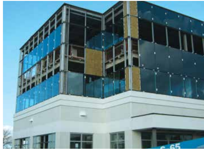
Developer Monterey Park used ROCKWOOL CURTAINROCK® insulation for its recently opened 75,000 sq. ft. commercial building in Brampton, Ontario.
