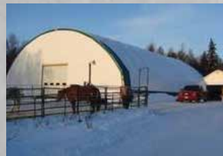
This building was “designed,” just not to the correct loading for the area.
