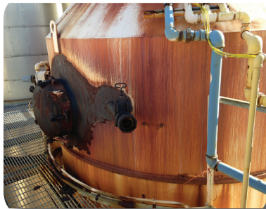
A severely corroded and unsafe combustion chamber
