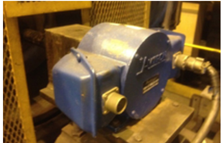
Figure 4B-Dual Output Pulse Generator installation
