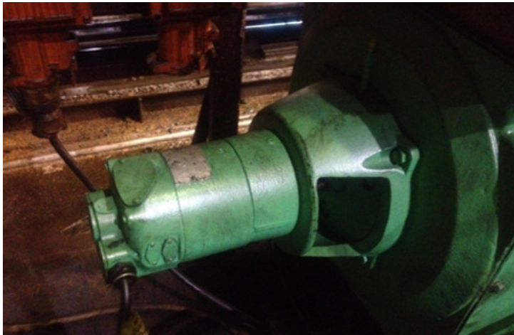
Figure 1-A General Electric BC46 Tach-Generator coupled to a DC motor
