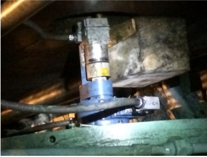
Figure 8 -Encoder and Overspeed mounted on Cold Mill
