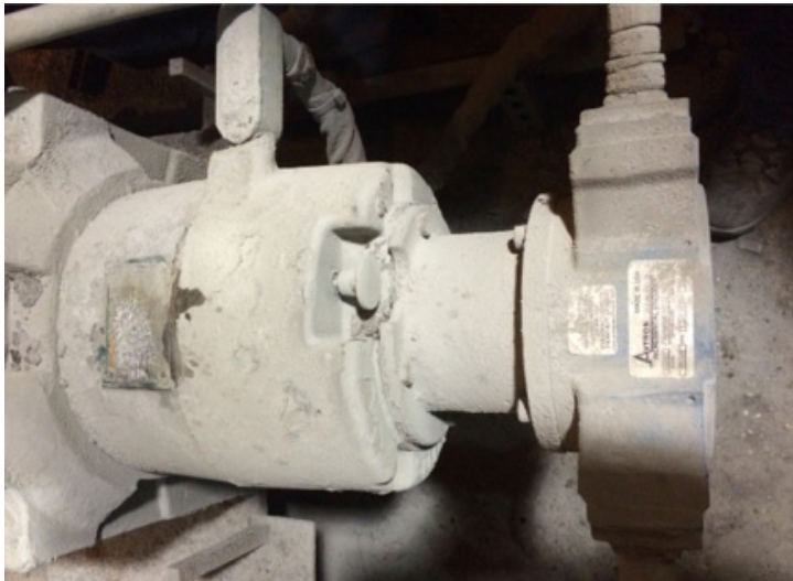
Figure 5 -Encoder mounted on Continuous Caster Brake
