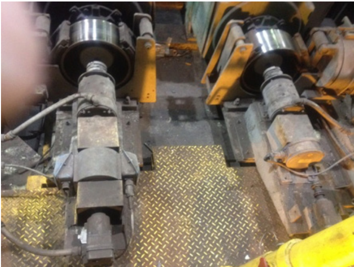
Figure 9 -Encoders mounted on Galvanizing Line
