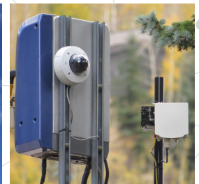
Siklu backhauls hybrid HD-CCTV, smart parking and public Wi-Fi in the Town of Vail, CO
