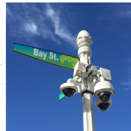
The City of Fort Myers selects Siklu's mmWave wireless for its Video Surveillance System
