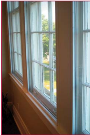
Climate Seal™ Acoustic Series window insert applied over historic wooden windows at the Mary O'Keefe Cultural Center. Ocean Springs, MS.
