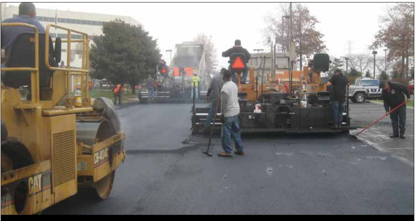
Brahney said one of his company's advantages is the amount of resources available. For this 4,000-ton mill and pave project for an office building, they were able to bring three pavers, six rollers and more than 20 workers.
