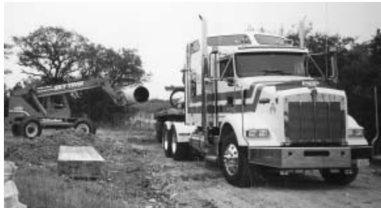
PEP Transportation arrives with pipe and fittings from QWP at one of three Natgun water construction projects in Texas.
