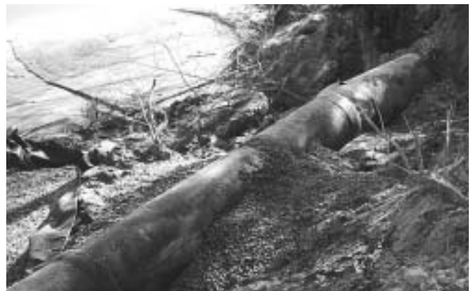
A portion of the 60' section of the washed out 36" sewer main on the banks of the Androscoggin River.
