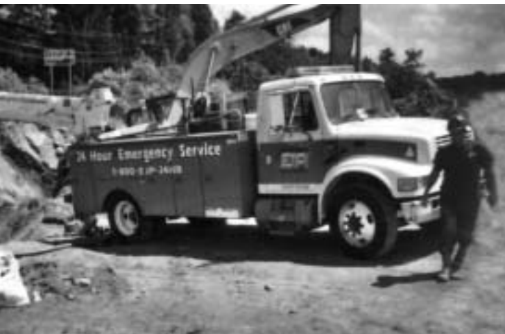
Brian Burns, EJP Technician, and service truck set up for installing 12" AFC Gate Valve.
