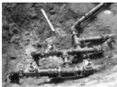
Four pipes converge into two.
