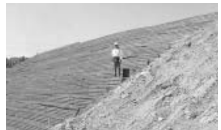
Cardi Corp's Benny Moriera stands on a portion of the Lincoln, RI highway project.
