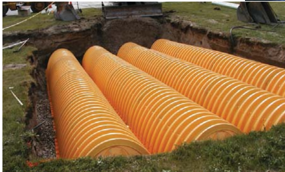
The Lake George drainage project comes together thanks to Team EJP Round Lake.
