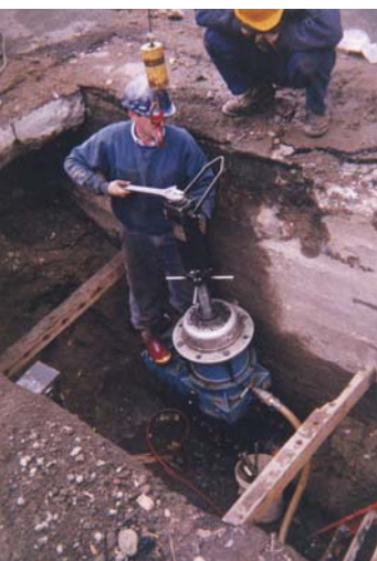
Ted Bragger of A.E. Bragger Construction monitors installation of an 8" insertion valve into an old cast iron main for the City of Pawtucket, RI.
