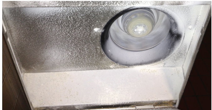
Fig. 2: Flour and dust buildup inside their previous competitor unit
