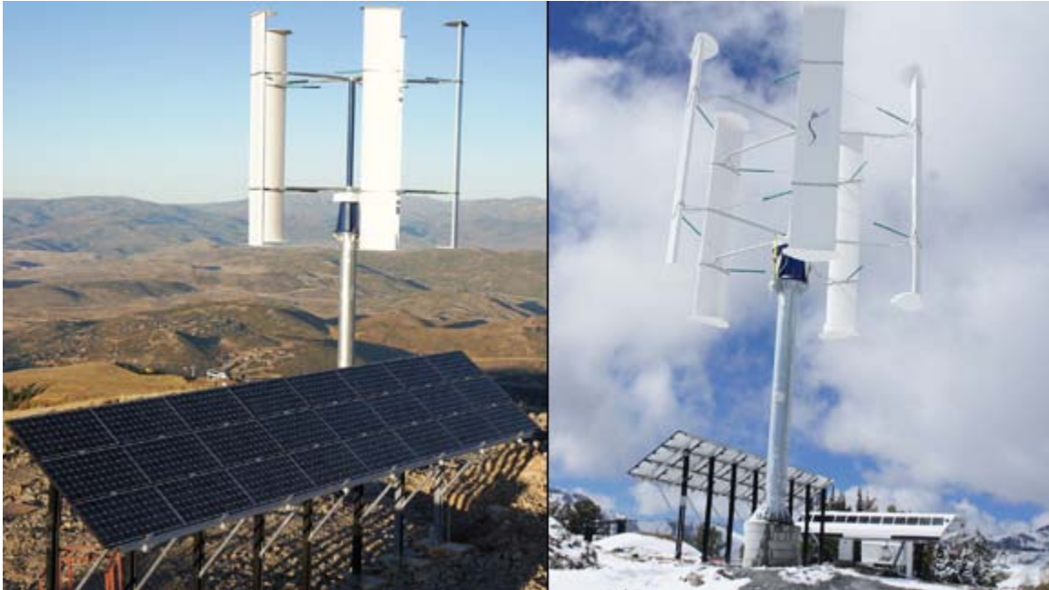
Summer and winter alternate views of Park City's wind and solar installation, which is located at the top of their Silverlode chairlift.
