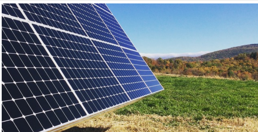
Innovative Vermont-made solar trackers are now providing emissions-free solar energy for The Alchemist's brewery, maker of wonderful Waterbury beer.
