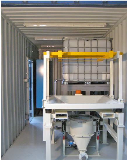
The mobile unit is housed in a 20ft/ 6m container
