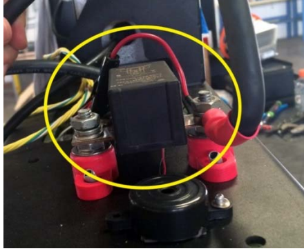
Figure 2: Latching relay inside the LiFT Pack.
