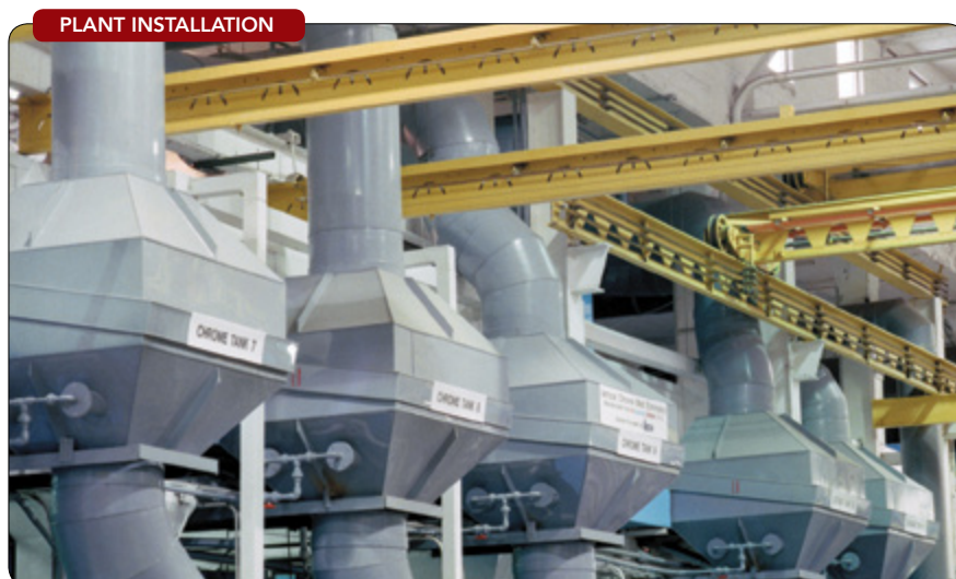
Figure 1. CPVC piping has a proven itself at plants for about 50 years; new formulations extend the applicability of the material.
