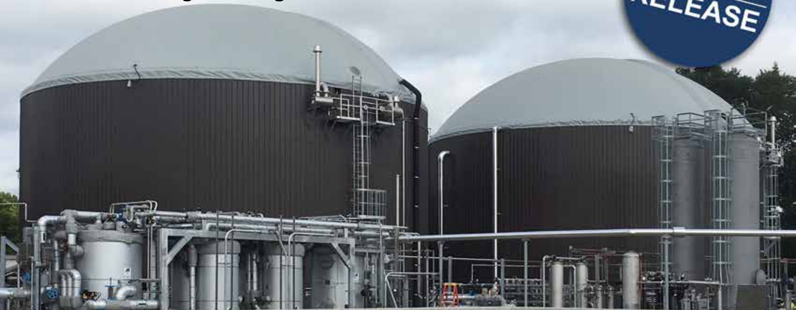
64ft. diameter x 40ft.SWH Digester units with gas collection DMR covers
