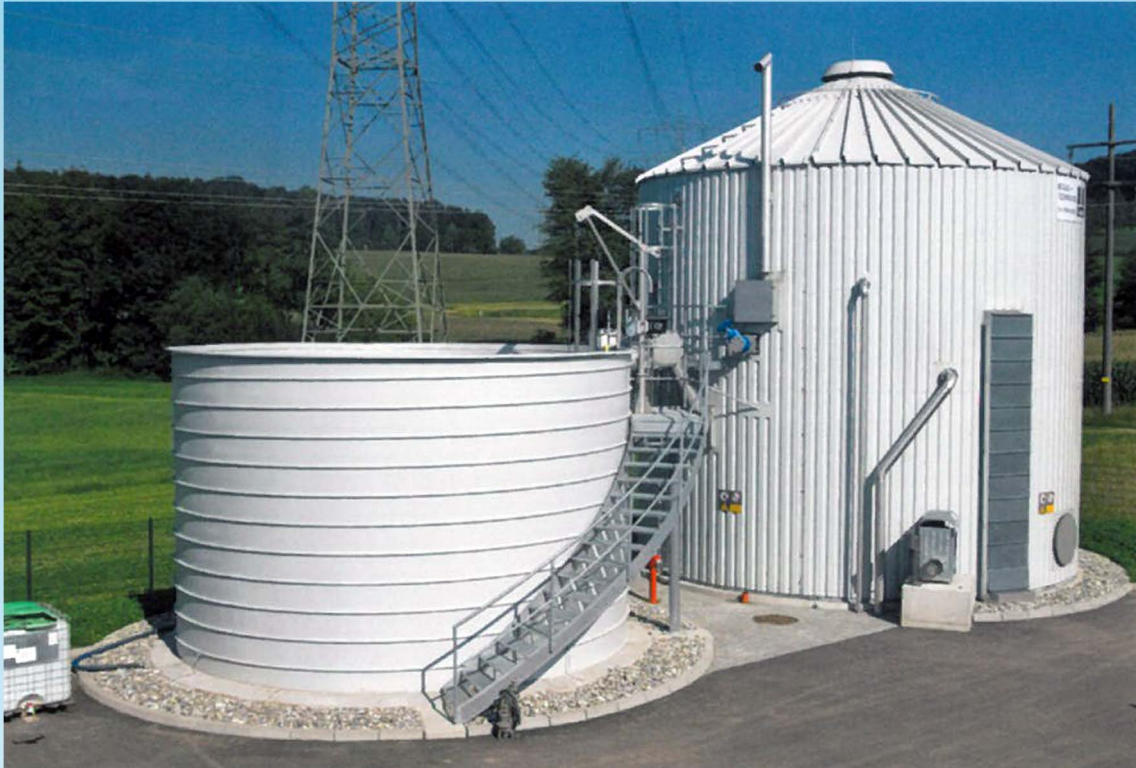
LIPP KomBio Reactor (60,000 gallons), sludge storage tank (35,000 gallons) on a municipal treatment plant
