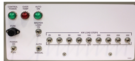
Remote Manual Control Panel shown.
