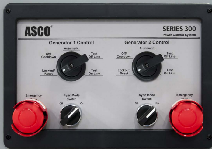
Figure 2: On this ASCO SERIES 300 equipment, setting the Generator Controls to “Lockout/Reset” and actuating and locking the Emergency Stop button is one method for isolating generators from the distribution equipment.
