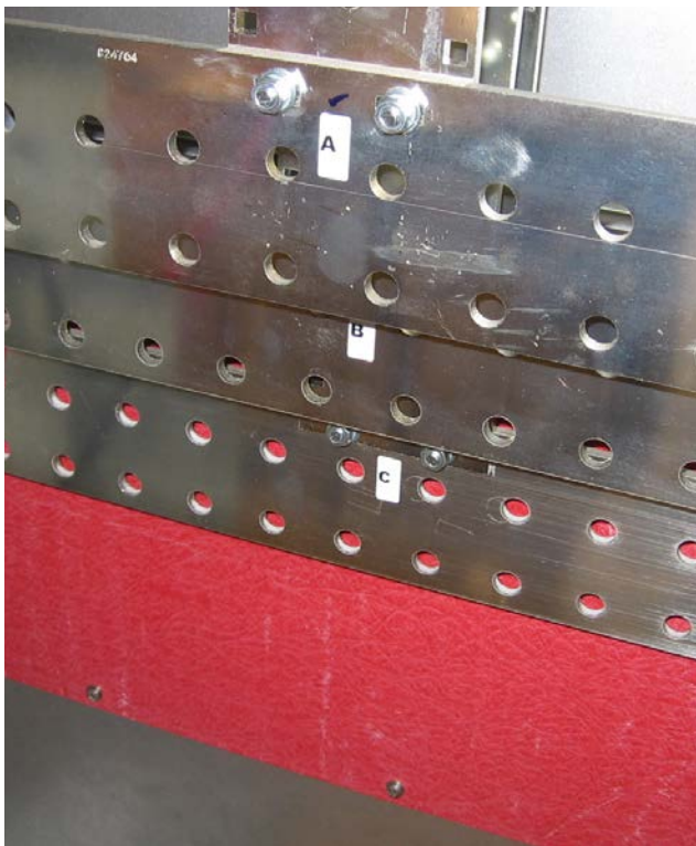
Figure 2: Bus Bar Connection Point.
