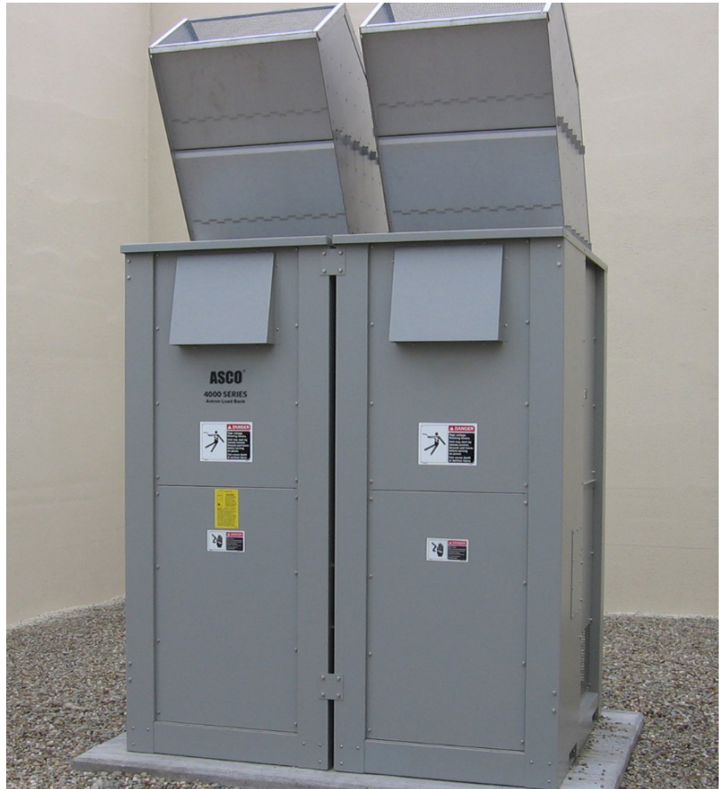
2000 kW Resistive Load Bank installed at a healthcare facility. (Photo courtesy of ASCO Power Technologies)
