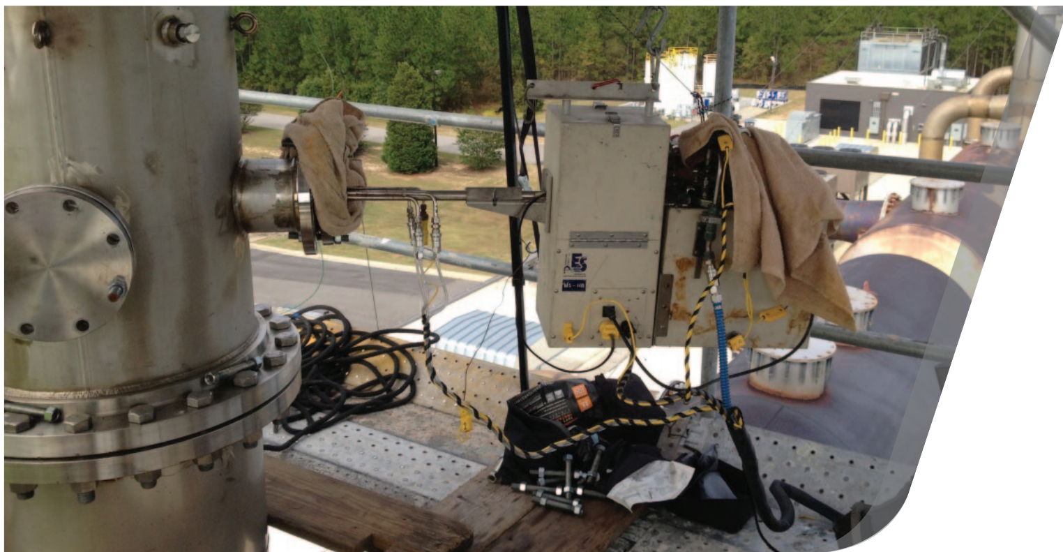
Figure 4: Probe aligned in stack
