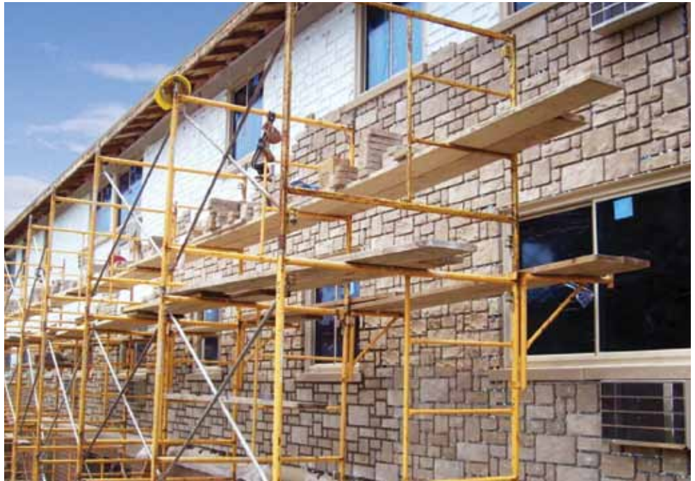
Continuous insulation helped a Wisconsin apartment rehab project win a government grant.
