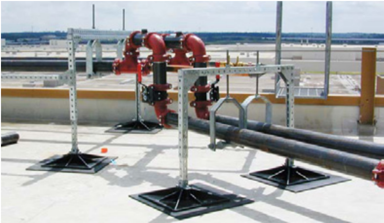
Multiple hanging HVAC piping
