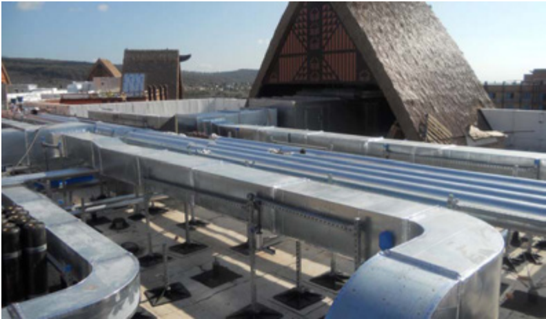
Duct and pipe support system with straight bracing
