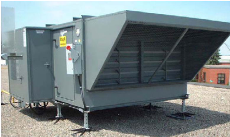
10 and 15-ton rooftop units with corner equipment supports raised 10" above roof
