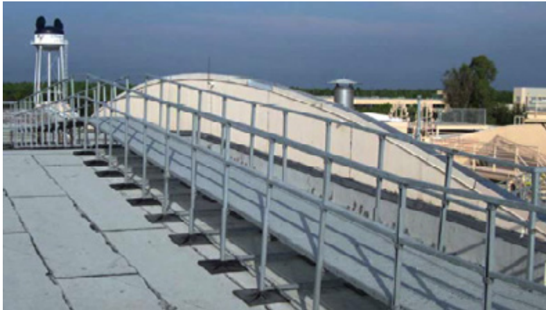
Walkway system, 4' wide, raised 30" off roof
