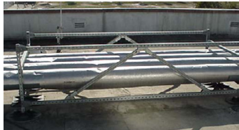
Enclosed pipe support system with k-bracing
