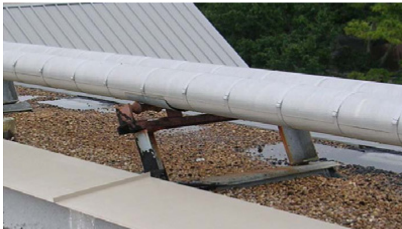
Inadequate design to manage thermal expansion & contraction
