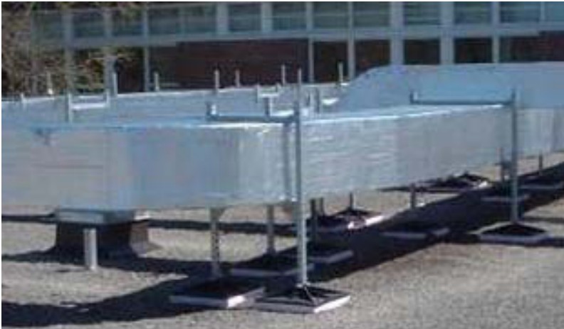
Enclosed duct supports
