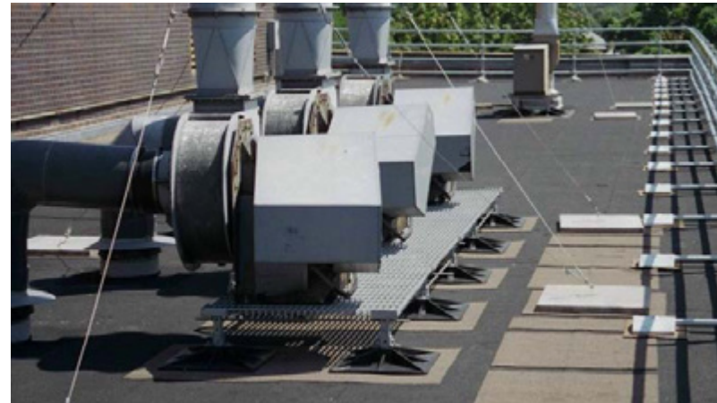
Equipment platform supports for blowers
