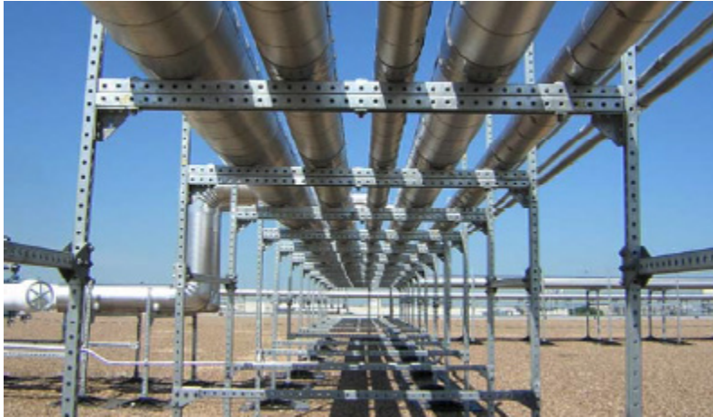
Open pipe support system with straight bracing
