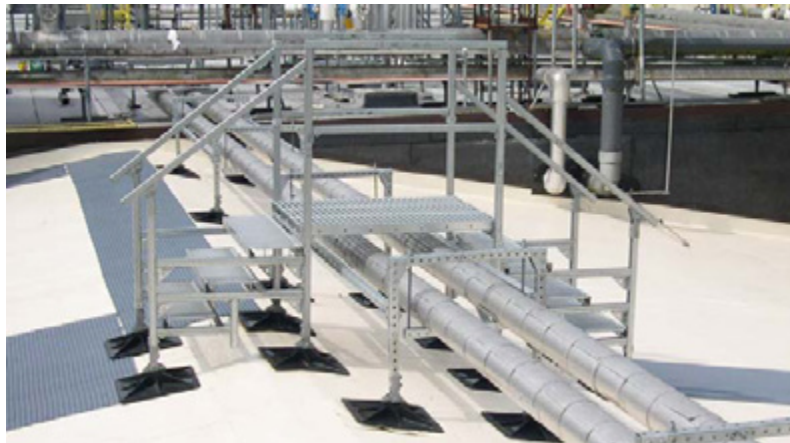
Leveling assembly attached to crossover and custom hanging supports with accessory bars on a sloped roof
