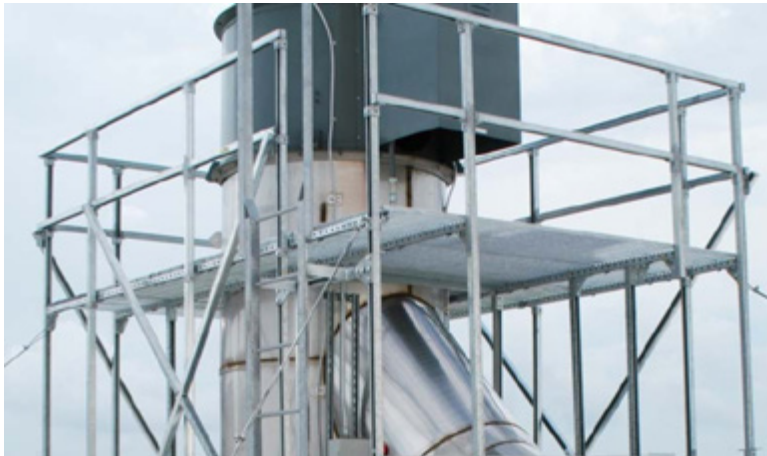
Tower access platform
