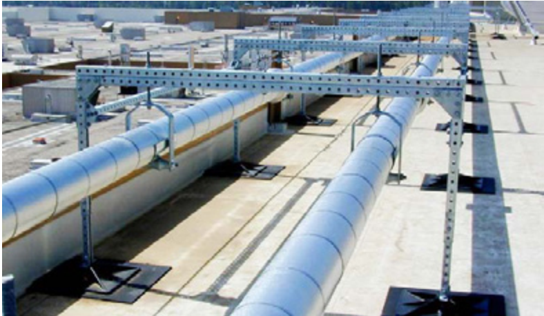
Multiple hanging gas piping
