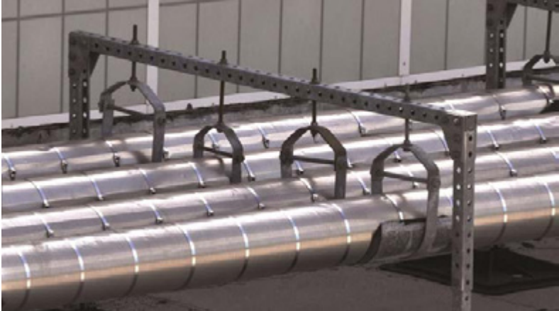
Multiple hanging gas piping
