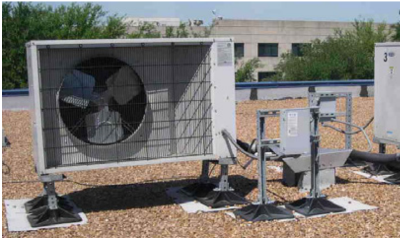
Rooftop blowers with corner supports and AC disconnect supports
