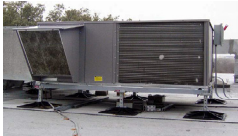
Multiple 10 and 15-ton rooftop units with center and corner equipment supports raised 10" above roof
