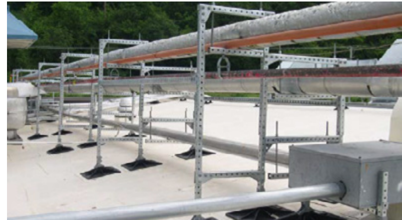
Enclosed pipe supports and custom hanging supports with clevis hanger and swivel assembly
