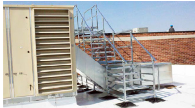
Crossover, spanning duct supports and 6' retaining wall
