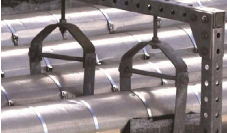
Pipe supports with clevis hangers
