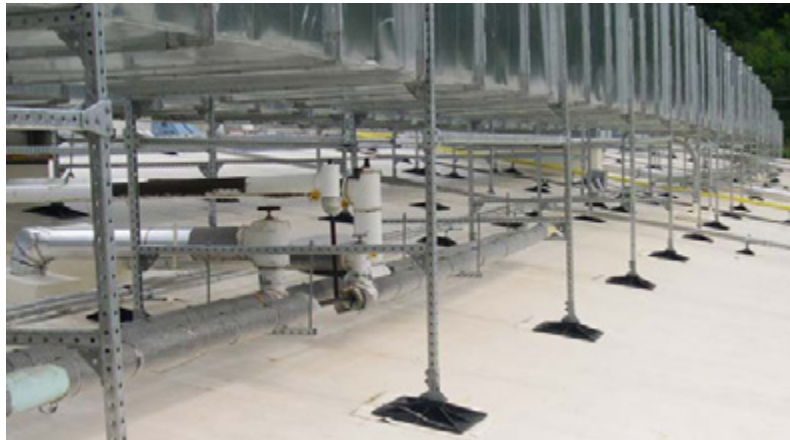
Open duct supports with swivel assembly, adjustable supports and pipe guides on sloped roof
