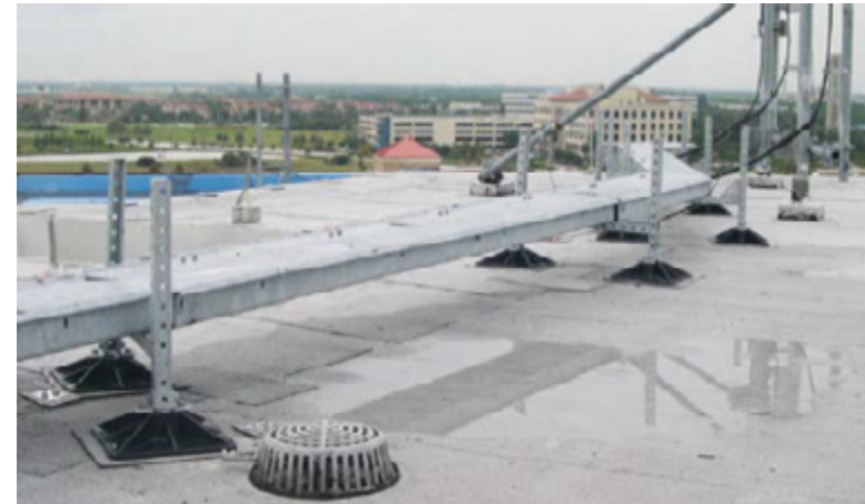
Cable tray raised 12" off roof
