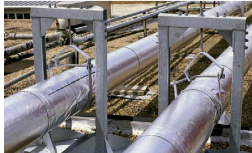
Inadequate design to manage weight
