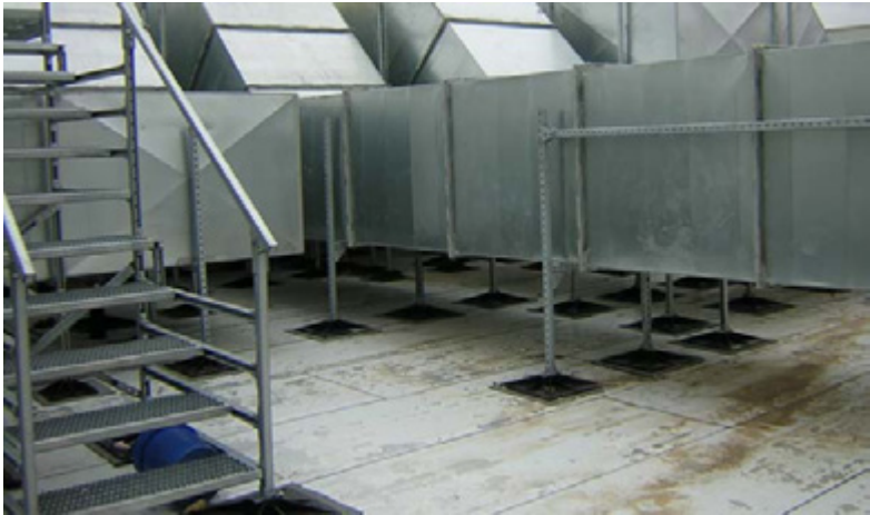
Open duct supports with straight bracing and crossover system
