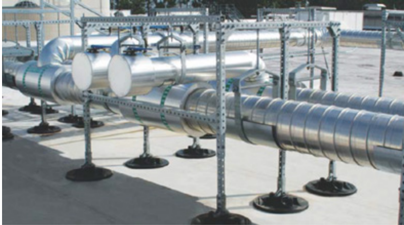
Multiple hanging gas piping with center leg support
