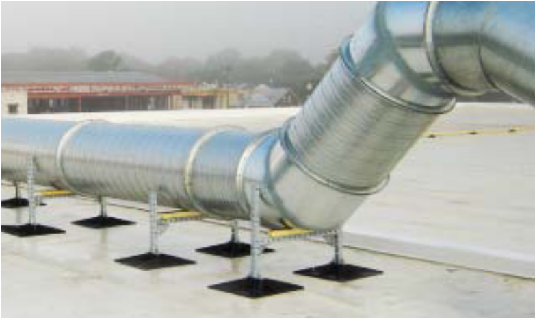
Open duct supports
