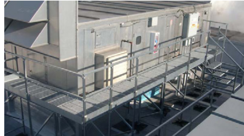
Walkway system with OSHA railing and stairs
