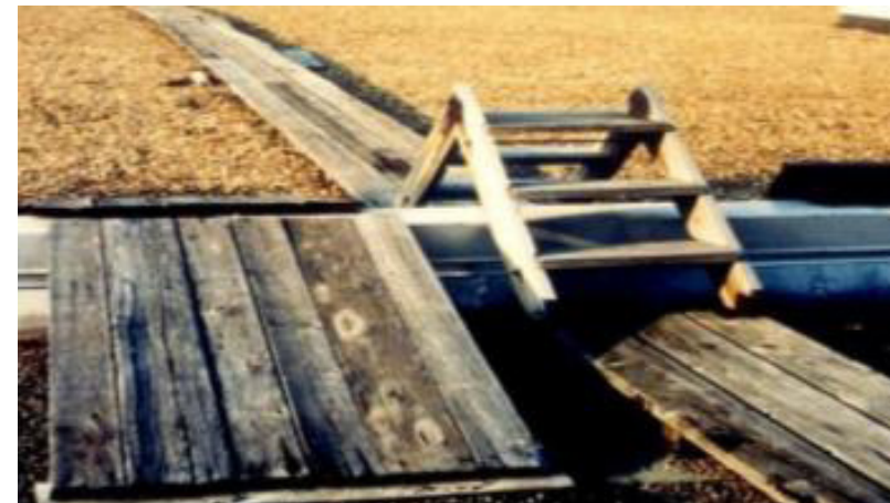
Inadequate walkway causing roof penetrations
