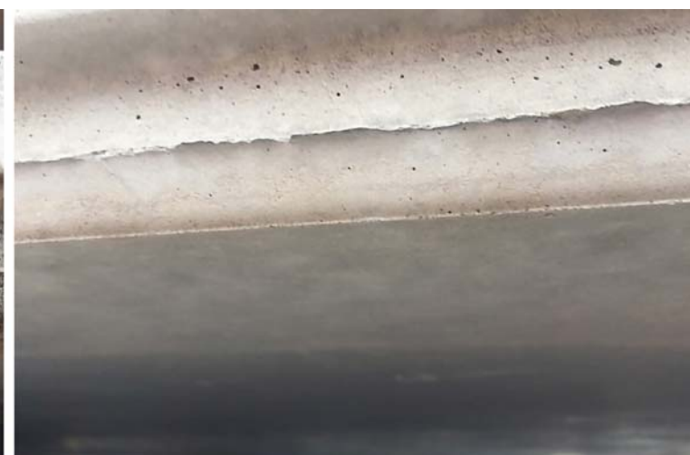
..... Stained concrete – left, before with over-application of mineral oil; right, after with vegetable oil release agent.
