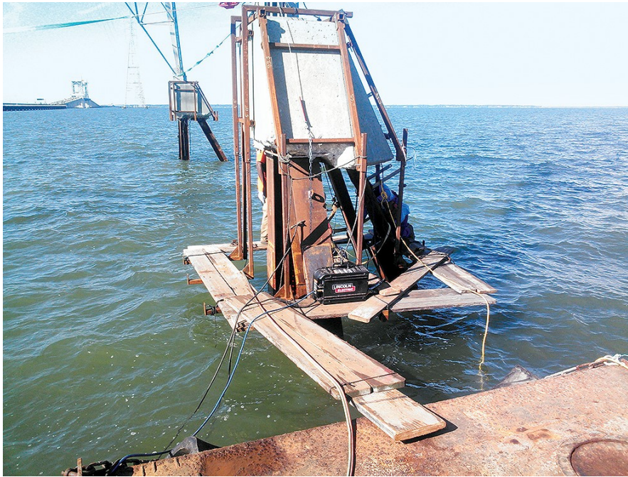
A portion of deteriorated H-pile is removed and a half H-pile replacement section is set into position.
