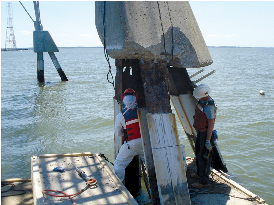
In preparing for H-pile section replacement, workers remove a portion of the concrete cap bottom and cut back portions of the existing encapsulation system.
