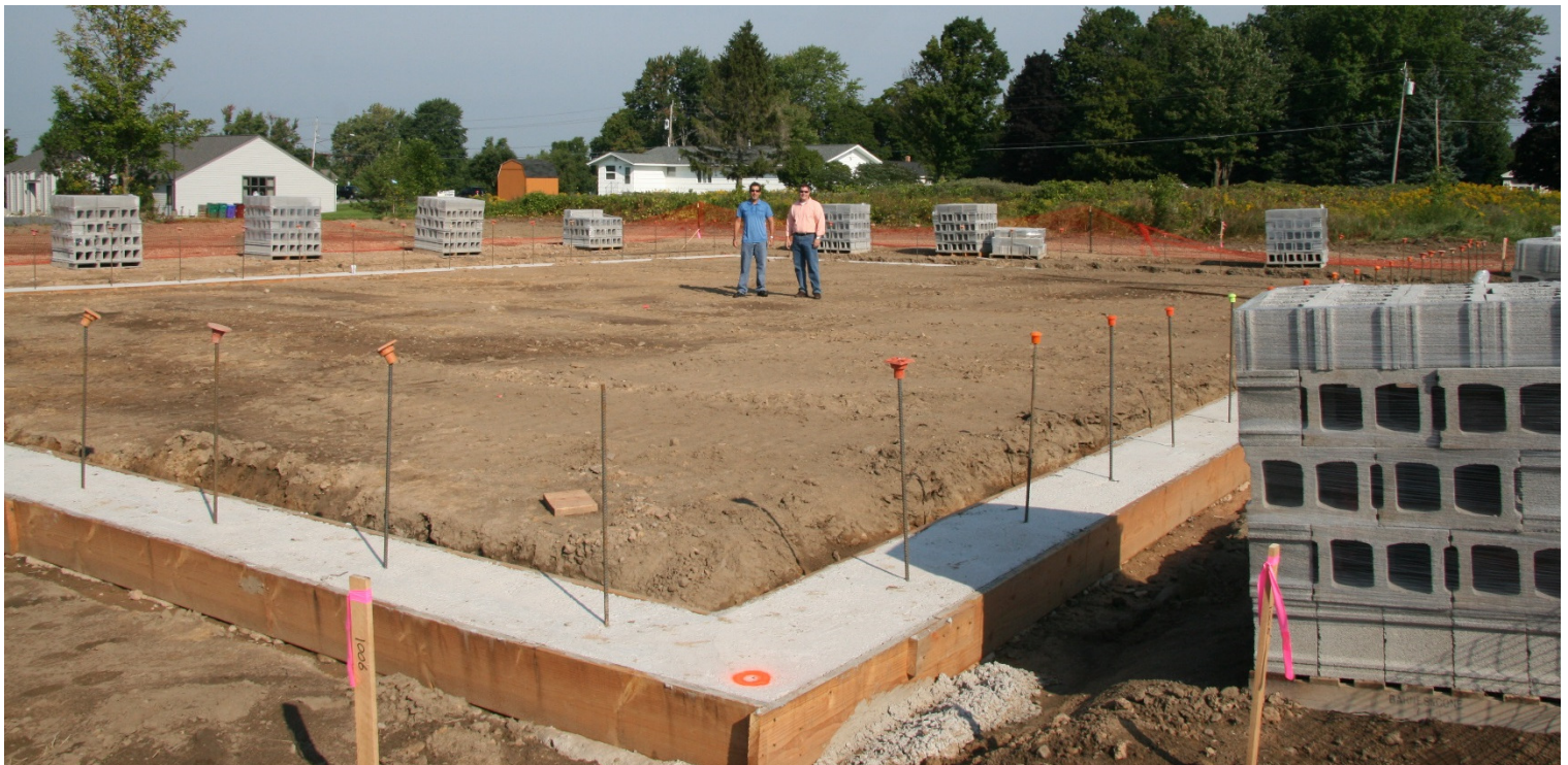
President/Owner, Phil Bova and VP of Operations, Tim Buckles stand in the construction area of the future facility on September 5, 2014.
