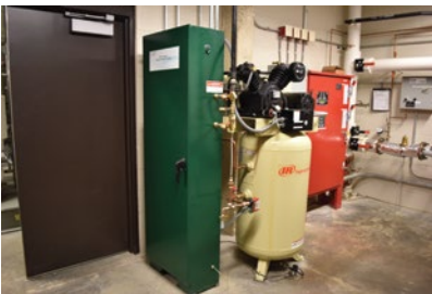
Nitrogen Generator installed in Riser Room
