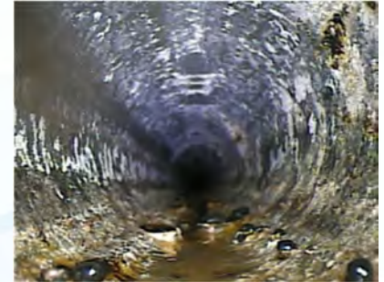
Corroded Galvanized Main
