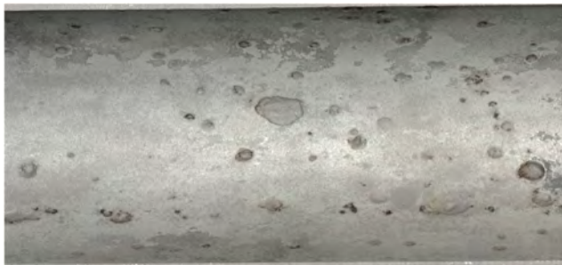
Under Deposit Accelerated Oxygen Corrosion
