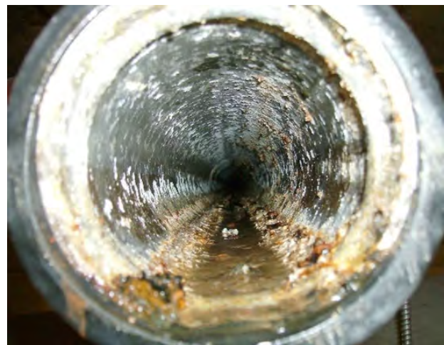
Corroded Galvanized Main with Trapped Water
