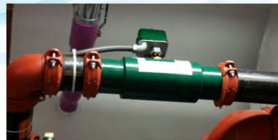
4 in. In-Line Detector installed in building
