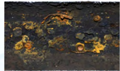
Corroded Branch Line
