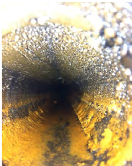
Corrosion from Trapped Air
