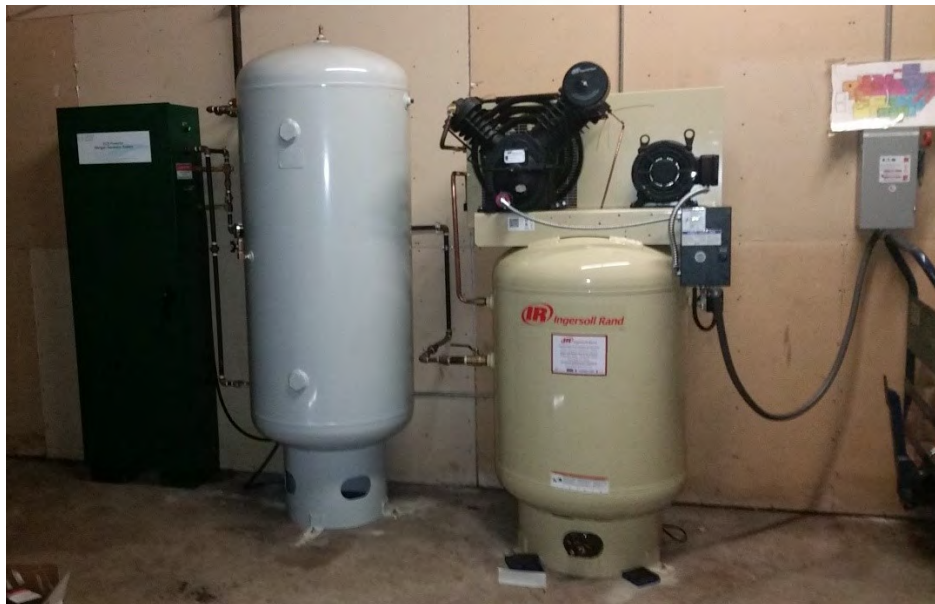
ECS Nitrogen Generator, storage tank, and air compressor feeding nitrogen supply
