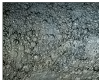
Under Deposit Accelerated Oxygen Corrosion
