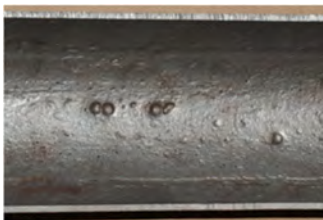
Oxygen Corrosion Pitting on Branch Line
