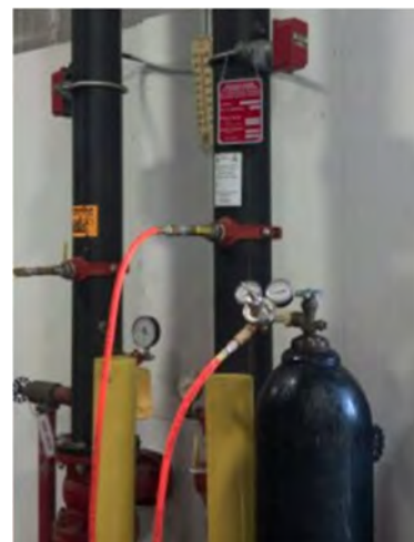
Pressurized Cylinders Provide Nitrogen Gas
